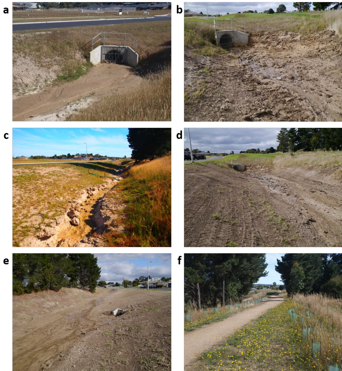
Figure 6. Pennyweight Gully. a shows the build up of sediment at the drain, that was subsequently cleared (shown in b). c–e show the straight, unvegetated stretch of gully. f shows a raised rail-trail bike and walking path to the east of the gully.
